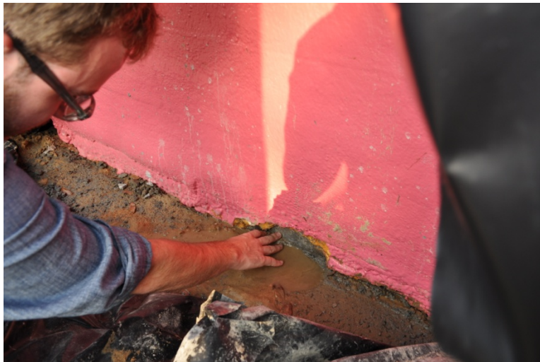
Fig. 4.19. PHOTO: Damage to test pod A: sealed block during the test fill.
