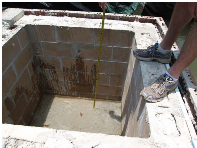
Fig. 4.39. PHOTO: Water seeping into test pod B2: cavity wall filled block, flood simulation 2.
